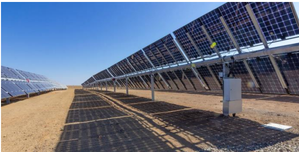
Figure 7 Bifacial photovoltaic systems
