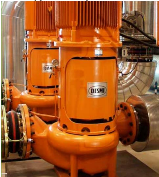
Figure 5: DESMI NSL300-415/E14 pumps fitted in the ballast system on board the ARSV Laurence M. Gould
